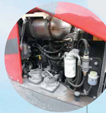
Above: A positive level of access is provided to the engine bay for inspection and routine servicing, and the fuel filter is easily reached for changing
